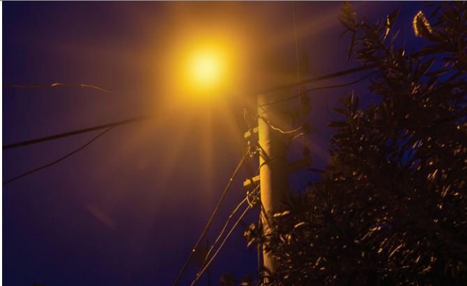
An example of the HPS streetlight (photo: The StressCrete Group)
